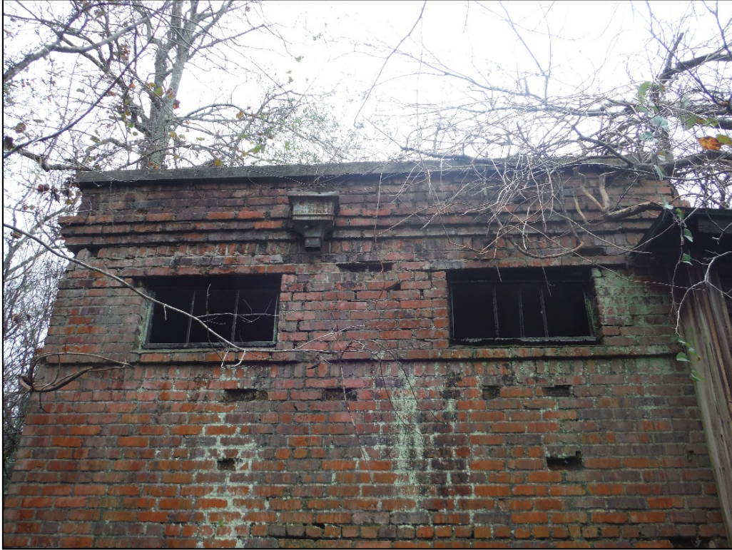
Figure 5. View of the Laurinburg Pump Station, window and brick detail, facing southwest.
