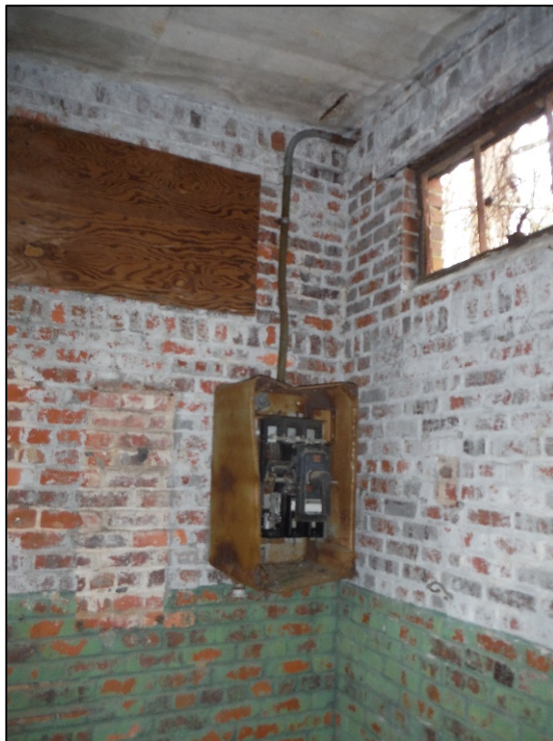
Figure 13. View of the Laurinburg Pump Station, interior, southeast corner.
