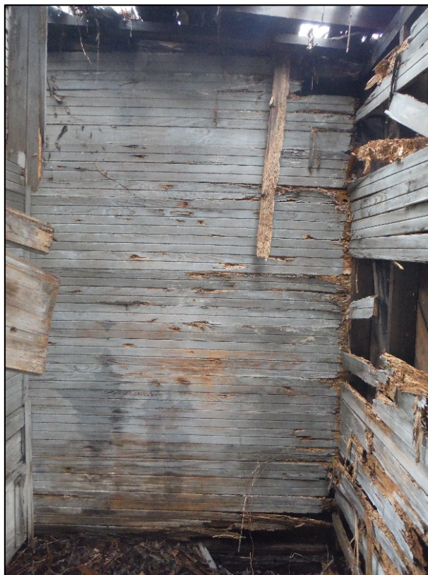
Figure 15. View of the Laurinburg Pump Station, interior of wooden extension, facing northwest.
